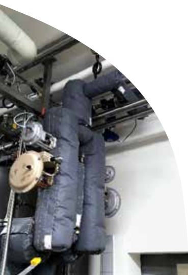
Steffca removable insulation padding mounted on pipes at CIP station
