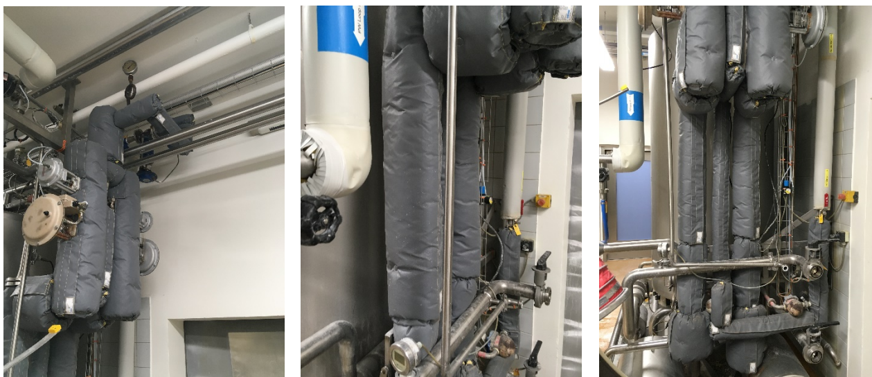
Steffca removable insulation padding mounted on pipes at CIP station.
